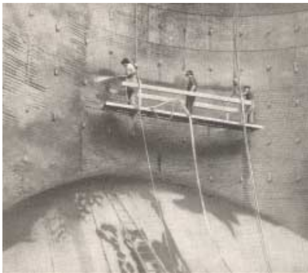
Figure 3. Restored, reinforced “Gunite” flue at American Smelting and Refining Co., Helena, Montana, 1924.
